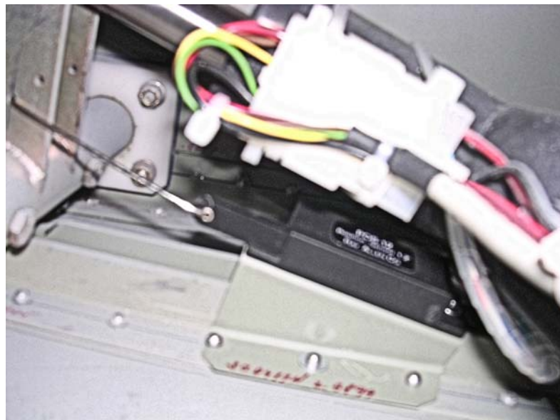
PICTURE 2 – Flaps sensor instalation
